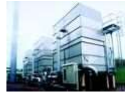
Cooling towers serving the four water-cooled chillers.
