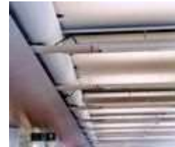
One of the central service bulkheads running through the office floor plates. The wing section partially conceals both the return and supply air ducts and the connections into the Termodeck planks.
